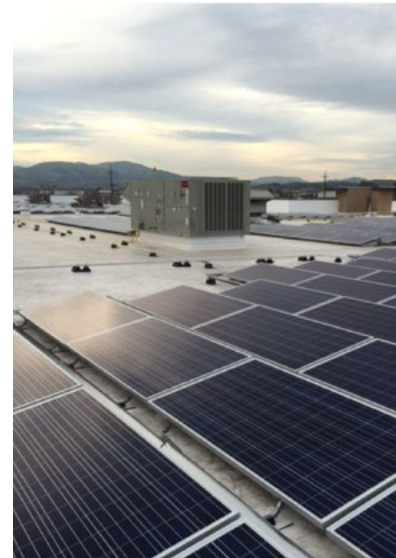
Solar panels on the roof of a Nordstrom Rack store.
